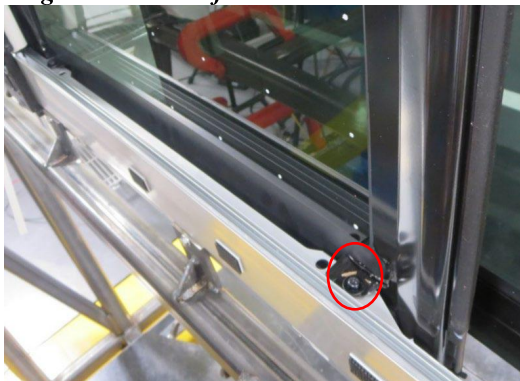
Figure 9. Panels attached to module using plastic brackets and glue along longitudinal edges.
